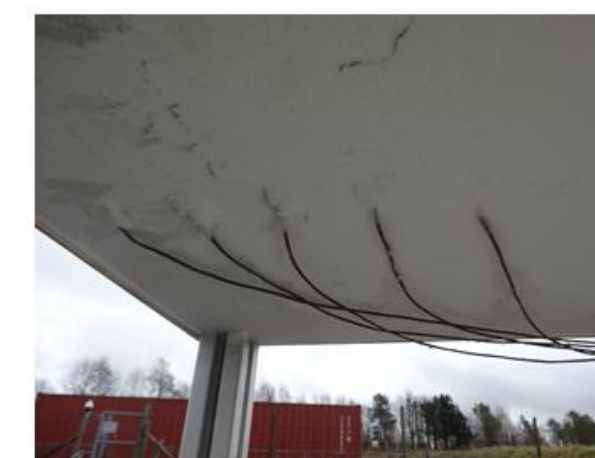
Steel plate underside after 200s release
